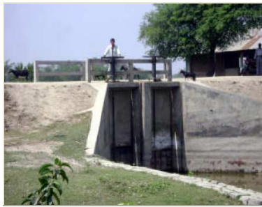
New Structure in IPSWAM
