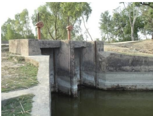
Figure 4.6: 2 vents sluice at Betibunia
