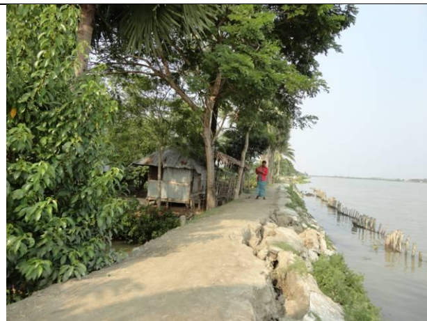
Figure 8: River erosion at Baro Banshbaria
