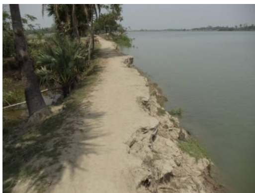
Figure 4.2: Daratana river bank erosion at Bashbari
