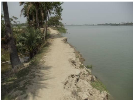
Figure 6.10: Embankment damaged at Bashbaria
