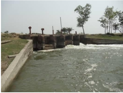
Figure 4.4: 6 vents sluice at Bara Bashbari
