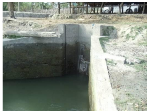
Figure 4.7: 1 vent flushing inlet at Mollikerber
